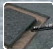
Spray all vertical edges (including manhole frame) with Ultracrete SCJ seal and tack coat
