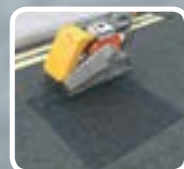
Ultracrete Instant Road Repair is compacted level with the existing surface. Apply Ultracrete Instaband ECO skid resistant overbanding tape if required
