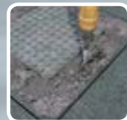
The picture frame is saw cut and excavated and the existing cover and frame removed
