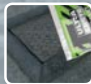
Apply Ultracrete Instant Road Repair cold lay asphalt concrete to a depth of approx 45mm, compacted to 30mm
