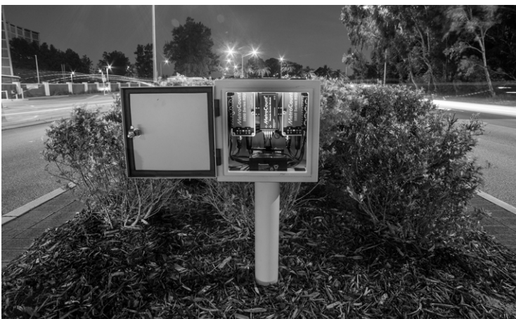
Counter, breakout board and modem in cabinet.
