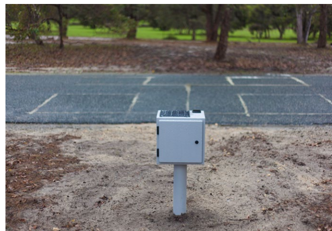
A freshly installed VL5810 on a low volume road.
