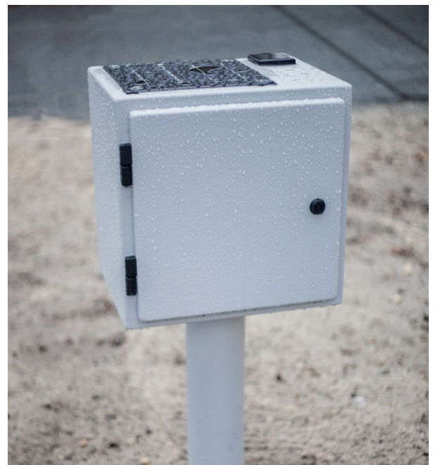
Weatherproof cabinet featuring 3G antenna and solar panel.
