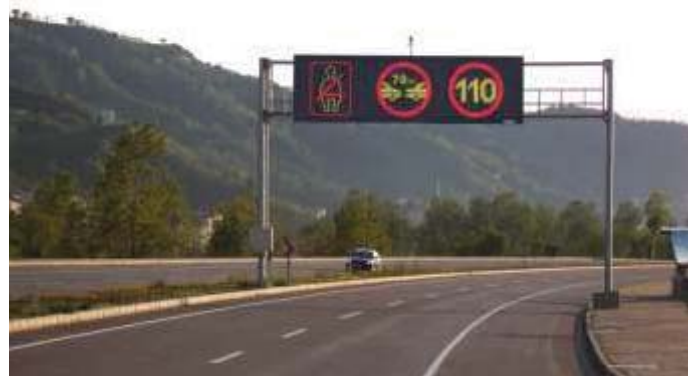
Blacksea Coast Road, Espiye Sarp Tunnels, VMS, TRABZON / 2009 Karadeniz Sahil Yolu, Espiye Sarp Tünelleri, VMS, TRABZON
