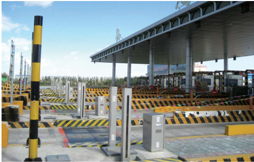
VanJee WIM system in toll station Guangdong China which consists WIM scale, infrared separator and deductive loop
