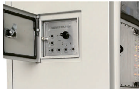
Manual panel of traffic signal controller
