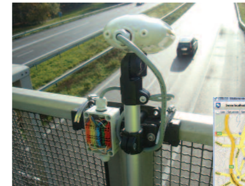
Traffic Data Collection, Incident Detection & Congestion Warning Sensor
