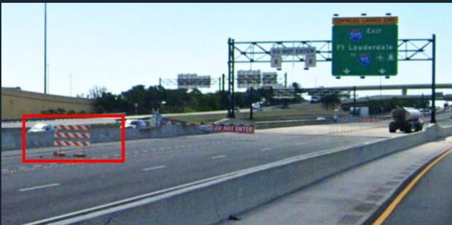
Supplemental barricades required to signal lane closure
